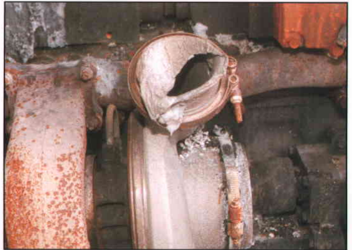
Photo 12 - Fire Damage Turbocharger Outlet Elbow (North Engine)
